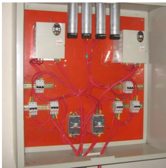
Fig.9.c Main control panel
