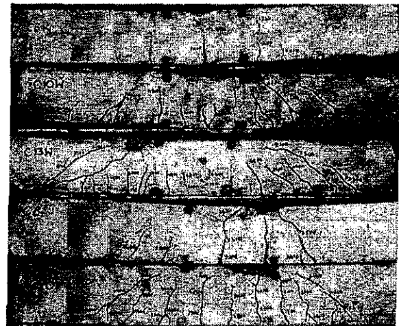
Fig. 5.a: Cracking pattern for control beams
