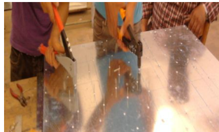
Fig. 8 Fixed rivets of TCP
