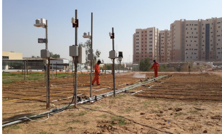
Fig 1: ET controllers after installation and set-up
