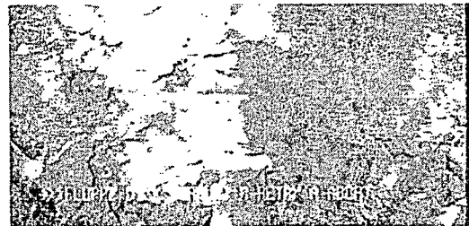
Fig. (8): CCTV Inside surfaced pipe showing fracture
