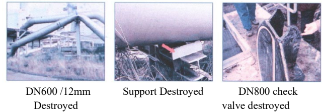
Figure 5. Damages caused by water hammer.
