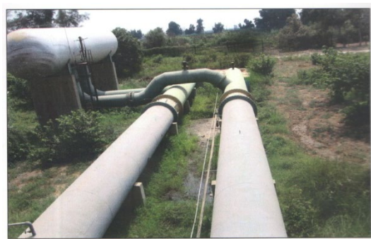
Figure 8. Irrigation pump plant photo.
