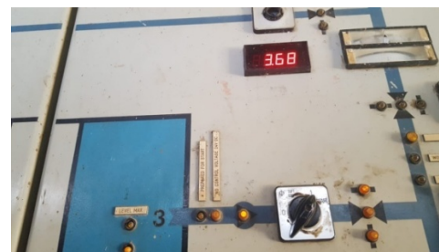
Figure 12. Main panel with pressure gauge indicator.
