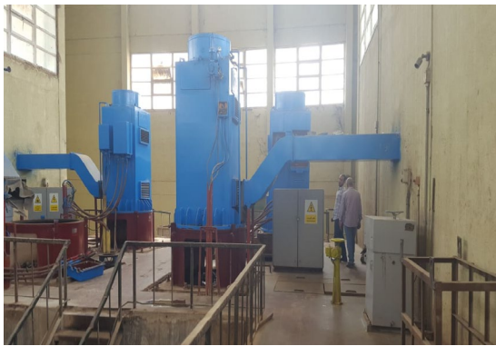
Figure 9. Irrigation pump plant photo.
