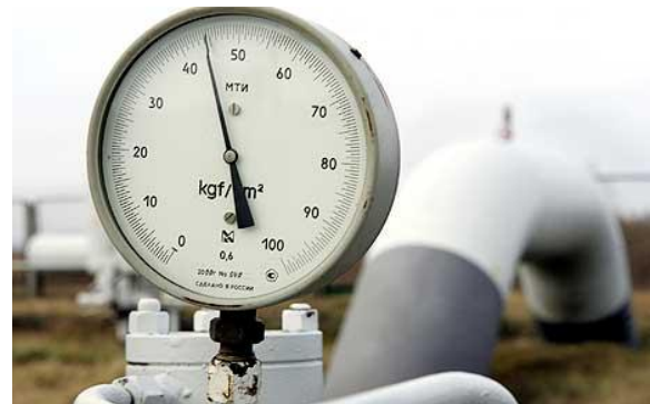
Figure 13. Main pipeline with pressure gauge.
